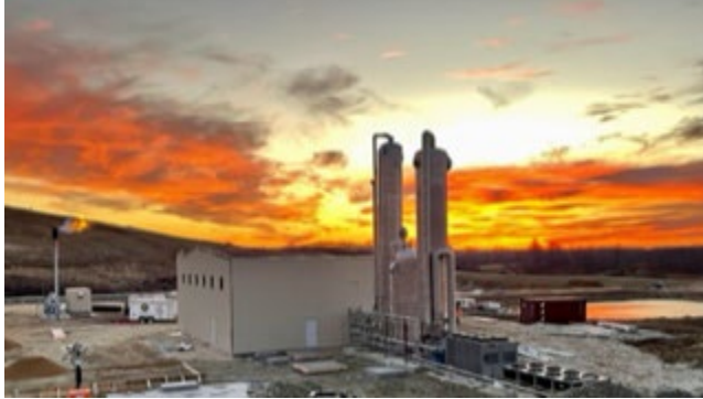
Photo Image 4: Eagle Ridge Landfill's Clean Energy Plant.
